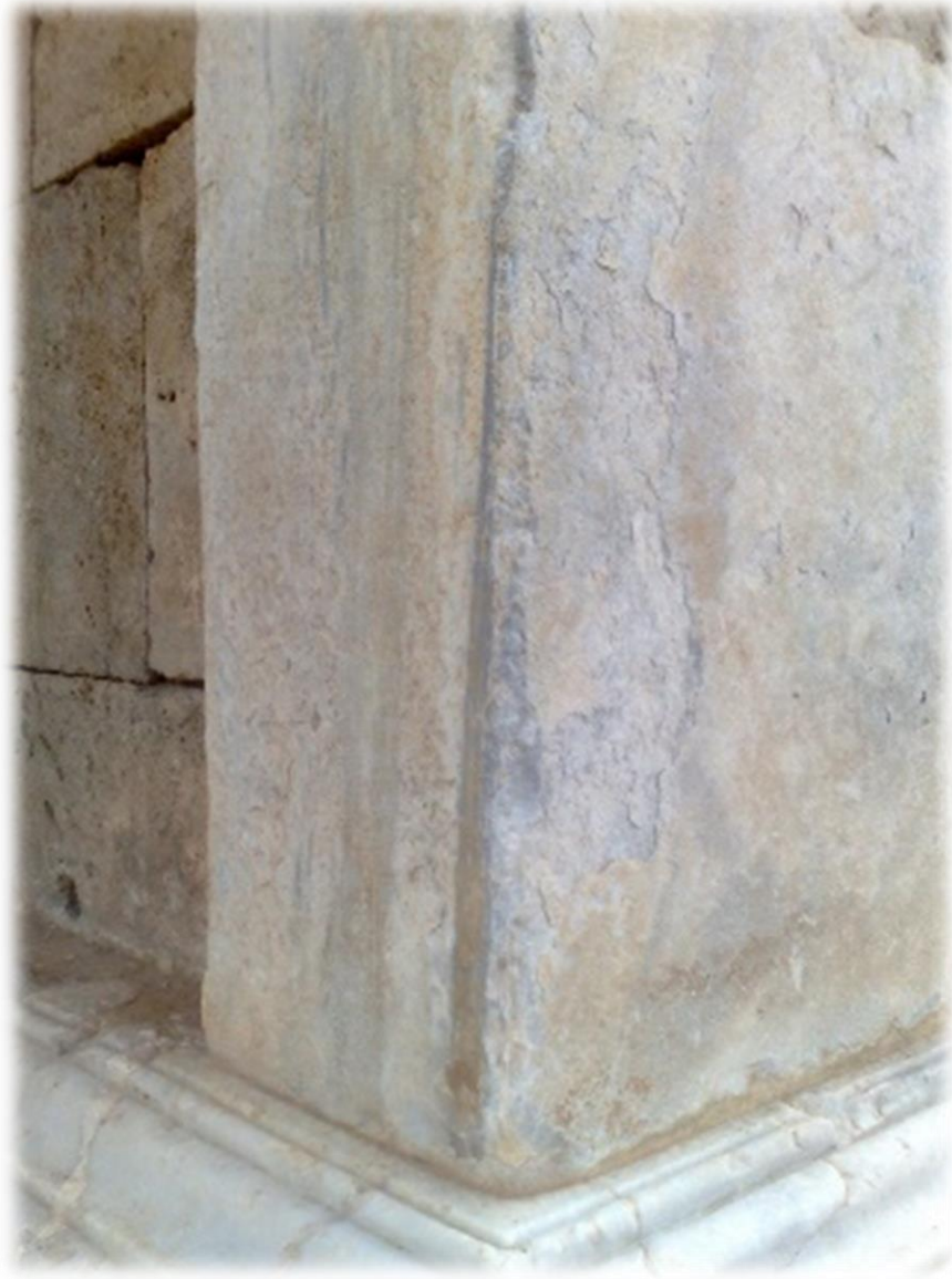
Figure (6): Erosion of a marble column forming crusts under the influence of air pollution.
