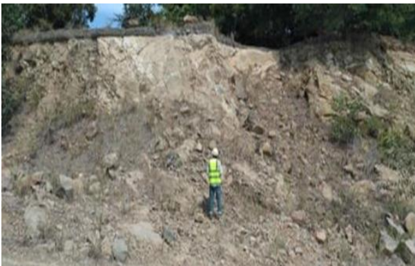
Figure (14): Shows how time affects a highly controlled parameter. Competent lithology (sandstone units) with high regulating factors weathers or erodes over time. Over a longer period, the decrease in sediment levels will have a significant impact on the rock, particularly where controlling factors are strong. Sediment loss occurs over longer time durations, despite the presence of strong controlling factors. The field photo was captured at Benoni Quarry, located in Sabah, Malaysia [1].
